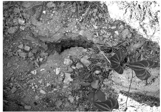
图2 郎漫公路上方山坡上的裂缝 Fig.2 Crack on hillside of Yunman Highway
