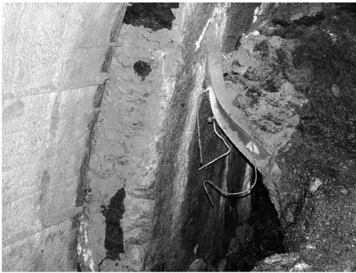
图1 云岭隧道ZK104+783处初期支护变形 Fig.1 Distortion in early days of support curve on ZK104+783 of Yunling Tunnel
