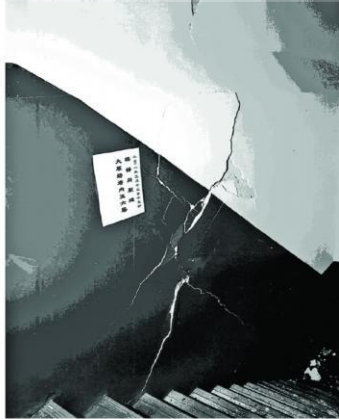
图3 六层楼梯裂缝 Fig.3 Cracks of 6th floor staircase
