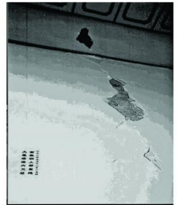
图5 七层西券洞上部开裂 Fig.5 Cracks of 7th floor west hole
