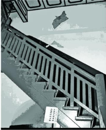
图2 五层东券洞上部开裂 Fig.2 Cracks of 5th floor east hole
