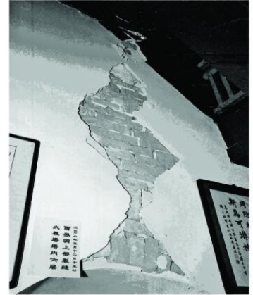
图4 六层西券洞上部开裂 Fig.4 Cracks of 6th floor west hole
